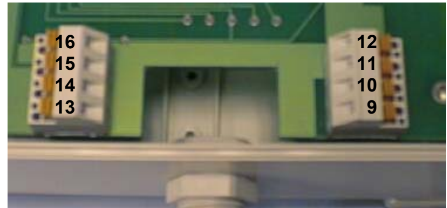
Terminal (located bottom right hand corner)
